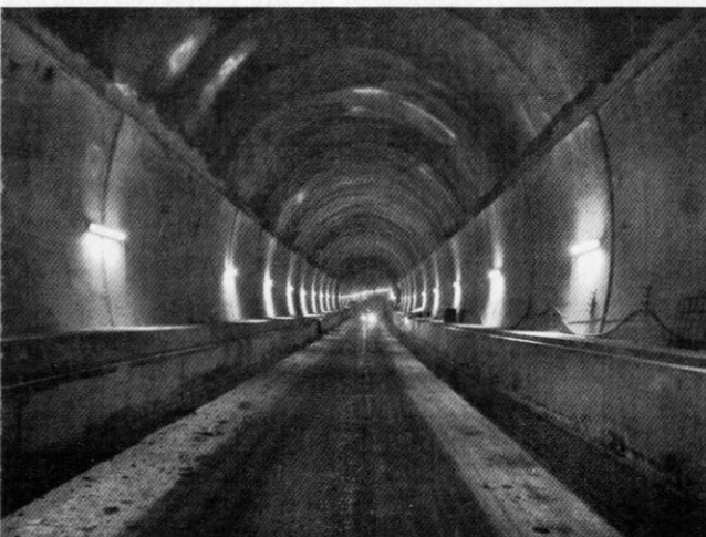
Construction of the tunnels was at an advanced state when Sub Brit visited in February 2010. Photo Nick Catford
